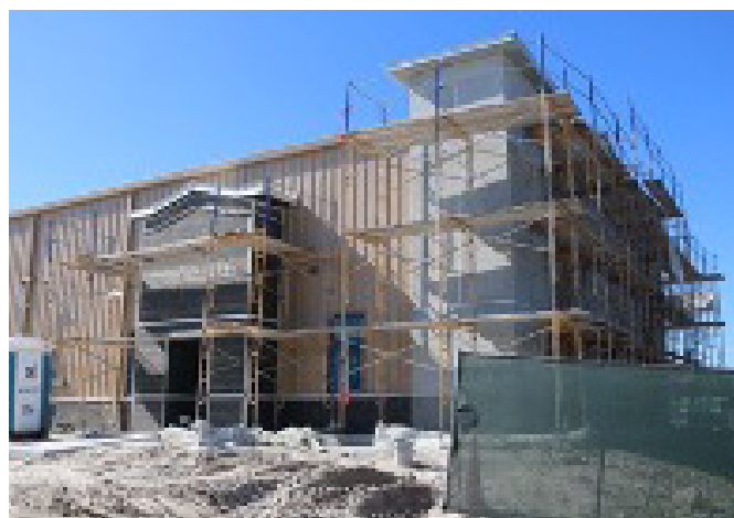
Sunbelt construction underway, commercial grant received in 2021, completion date extended to July 2023
