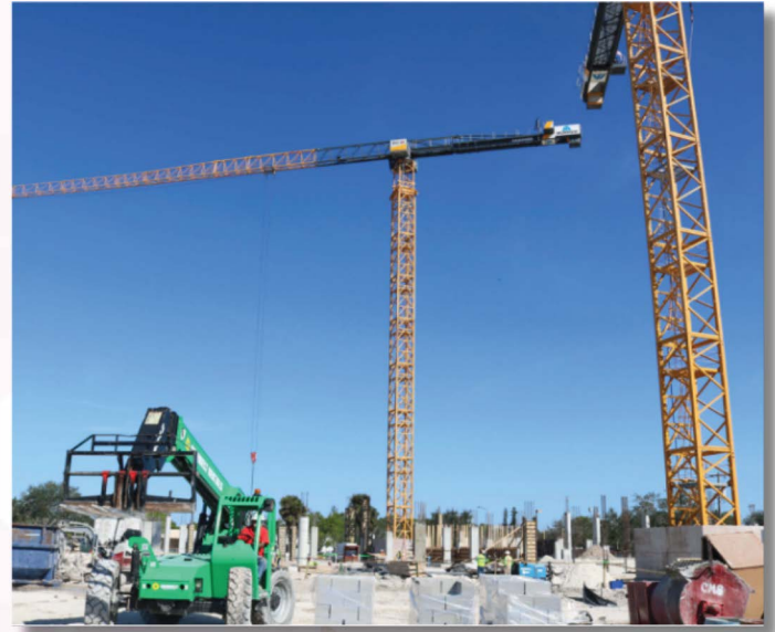
Cranes in operation as the initial phase of construction begins for Ascent
